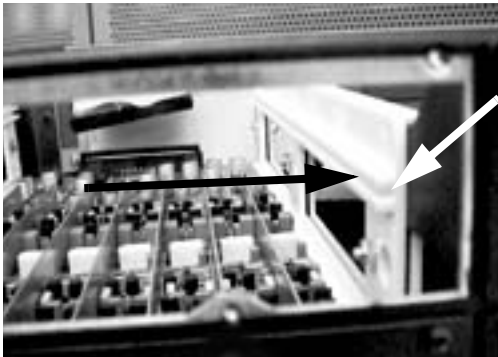
Example of an empty bay. Note guide rails along the inside edge
